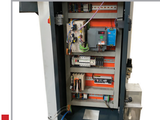
Elektik panosu Electric panel
